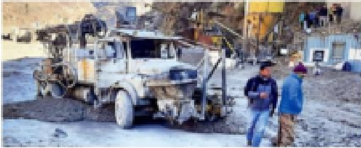
Locals inspect the site near damaged Dhauliganga hydropower project at Beni village, on Sunday
